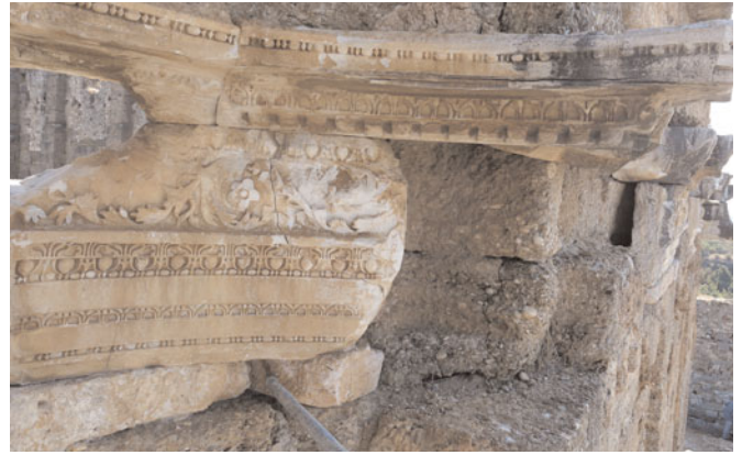
The entablature of the central niche, revealing the row of undecorated limestone blocks wedged in underneath the entablature and the conglomerate ashlars of the back wall partially cut back to receive the entablature
